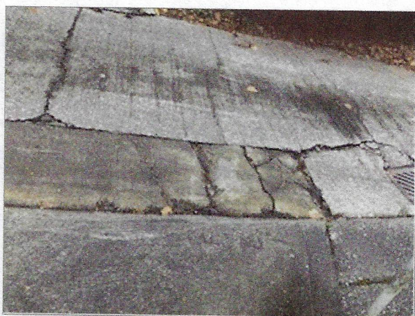
Exhibit 1: Distressed Pavement from Waterline Repair
