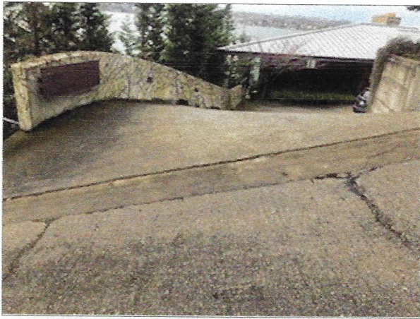
Exhibit 2: Driveway to Paring Apron, Note Hump.
